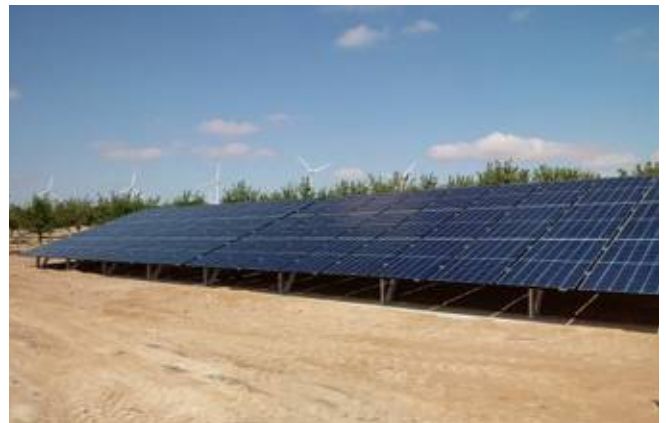
Bombeo solar Juan Vallado, Belchite
